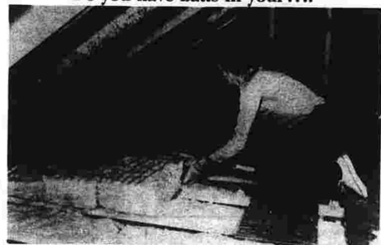
BATTS IN THE ATTIC AREN'T ALWAYS A NUISANCE. In the case of fiber glass insulation batts, they can be a life-saver, or at least an energy-and-money-saver. This homeowner is installing a double layer of six-inch fiber glass batts to bring his attic insulation up to a level of R-38 (12 inches); this is the recommended R-value of colder areas of the country according to the CertainTeed Home Institute. When he's done, he can sit in the comfort of a warm home knowing that he'll be saving heat and money for as long as he lives there.
